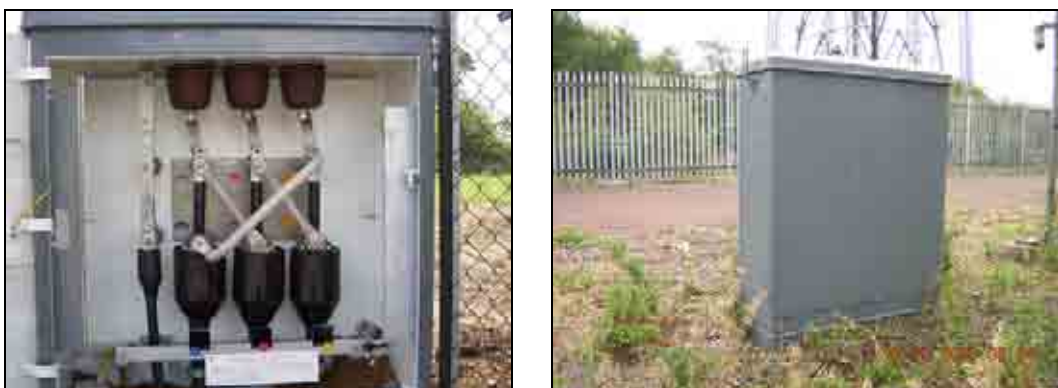
Plate 3.2 A typical cross-bonding link pillar
