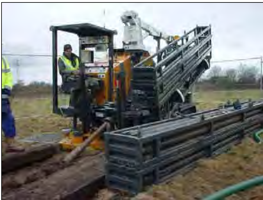
(photograph courtesy of Balfour Beatty Power Networks Ltd.)
