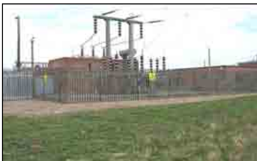
Plate 8.2 Existing EDFE substation
