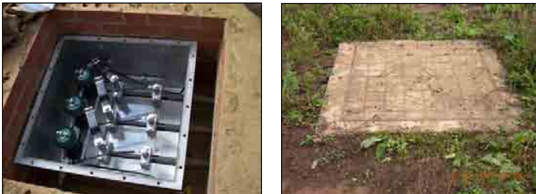
Plate 3.1 A typical cross-bonding pit link box and manhole
